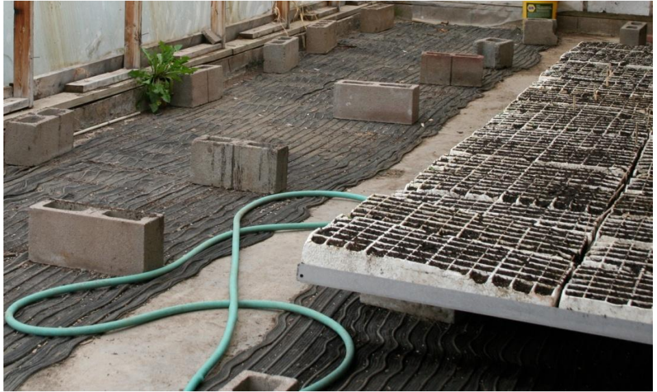
Rubber germination mats resting over concrete are connected to a 40-gallon water heater; hot water hoses alternate with hoses for transporting cooler water to the heater.
